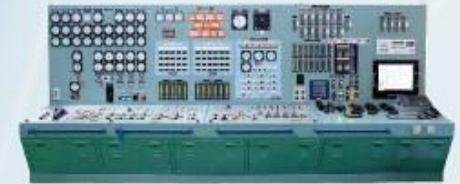
▲ Valve Remote Operation System Control Console
